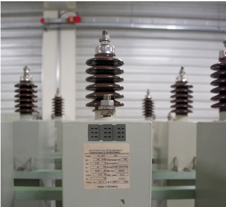
Capacitor Bank Monitoring
