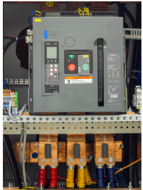
Circuit Breaker Monitoring
